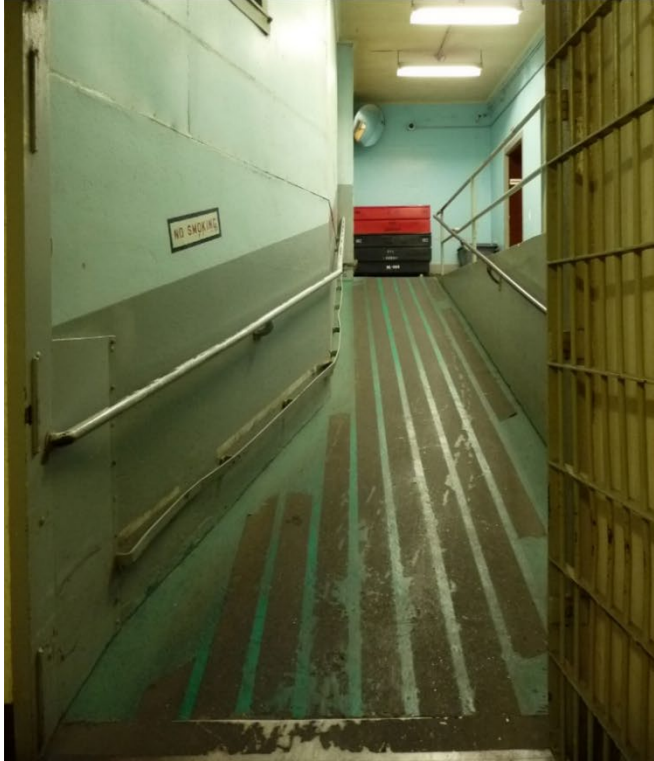
The Oregon State Penitentiary ramp to shower area is steep and creates accessibility issues.
