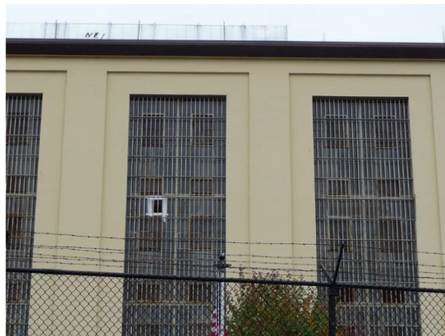
Old broken and poorly insulated windows at State Penitentiary offer little protection from extreme temperatures. Source: Auditor photo taken during a site visit.
