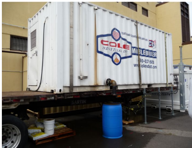
At the Oregon State Penitentiary, a temporary boiler costs $100,000 per month to operate. Source: Auditor photo taken during a site visit.
