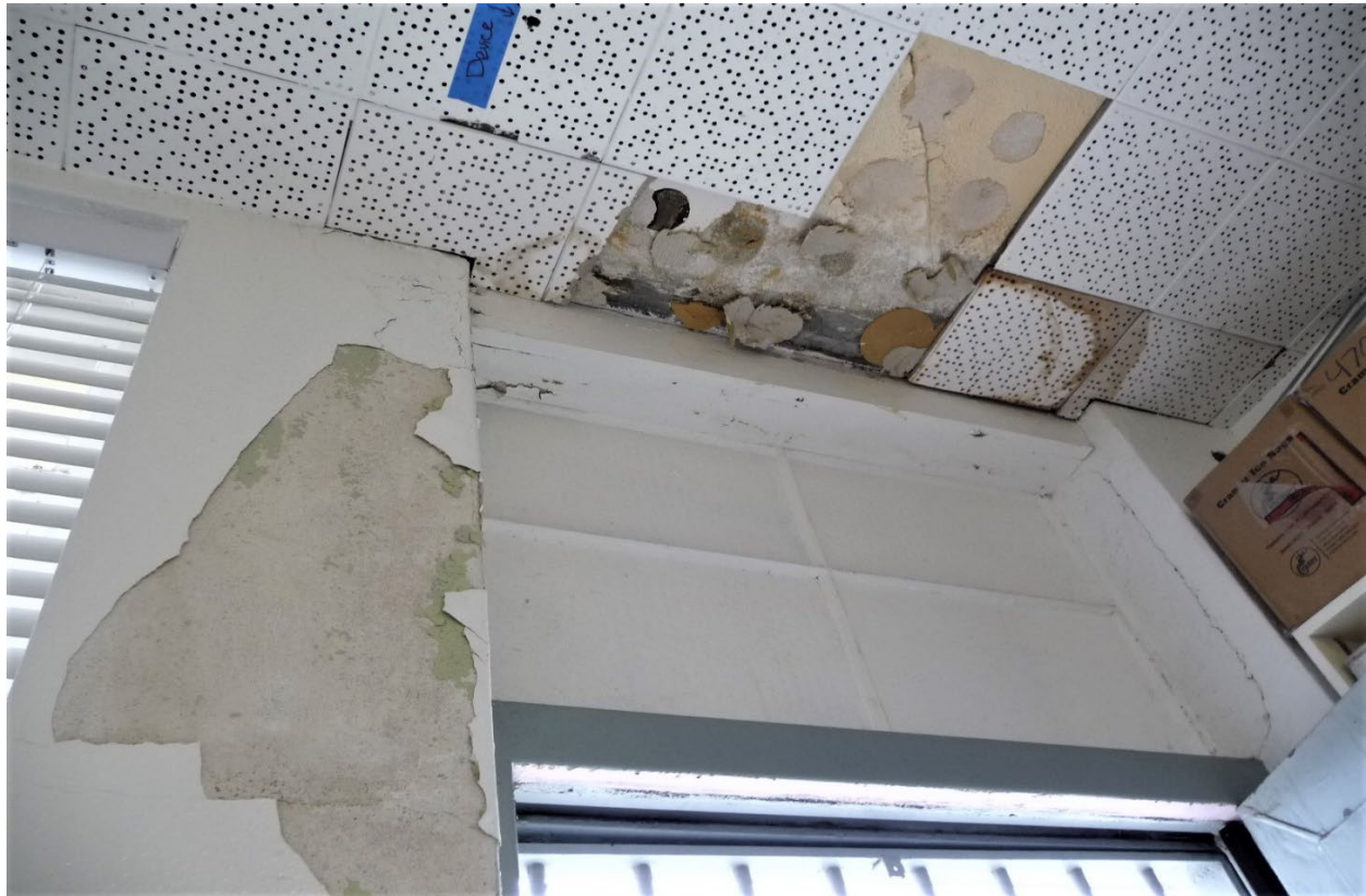
Asbestos tiles, chipped lead paint, mold, mildew and water damage appeared throughout the Oregon State Penitentiary. Source: Auditor photo taken during a site visit.
