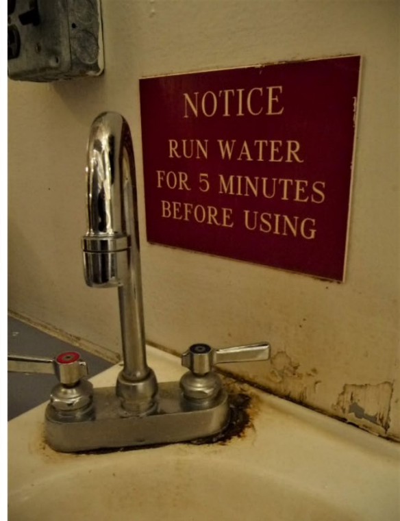
State Penitentiary Old pipes are gradually being replaced because of water quality and safety issues.
