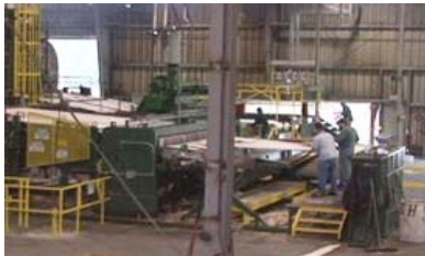
A 2010 SRF forgivable loan contributed to The Murphy Company’s refurbishment of a plywood mill in Rogue River.
